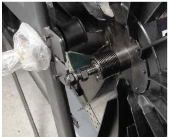
Fan shaft removed from frame bracket and Drive Belt
